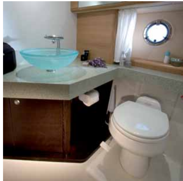
guest's wc and shower room - toilette ospiti
